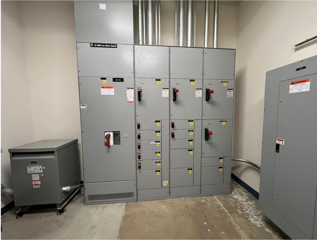
Figure 7 - Motor Control Center MCC15D
