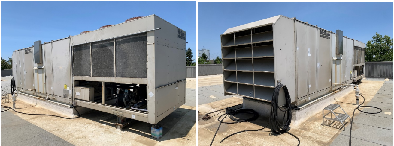
Figure 4 - Rooftop DOAS Unit
