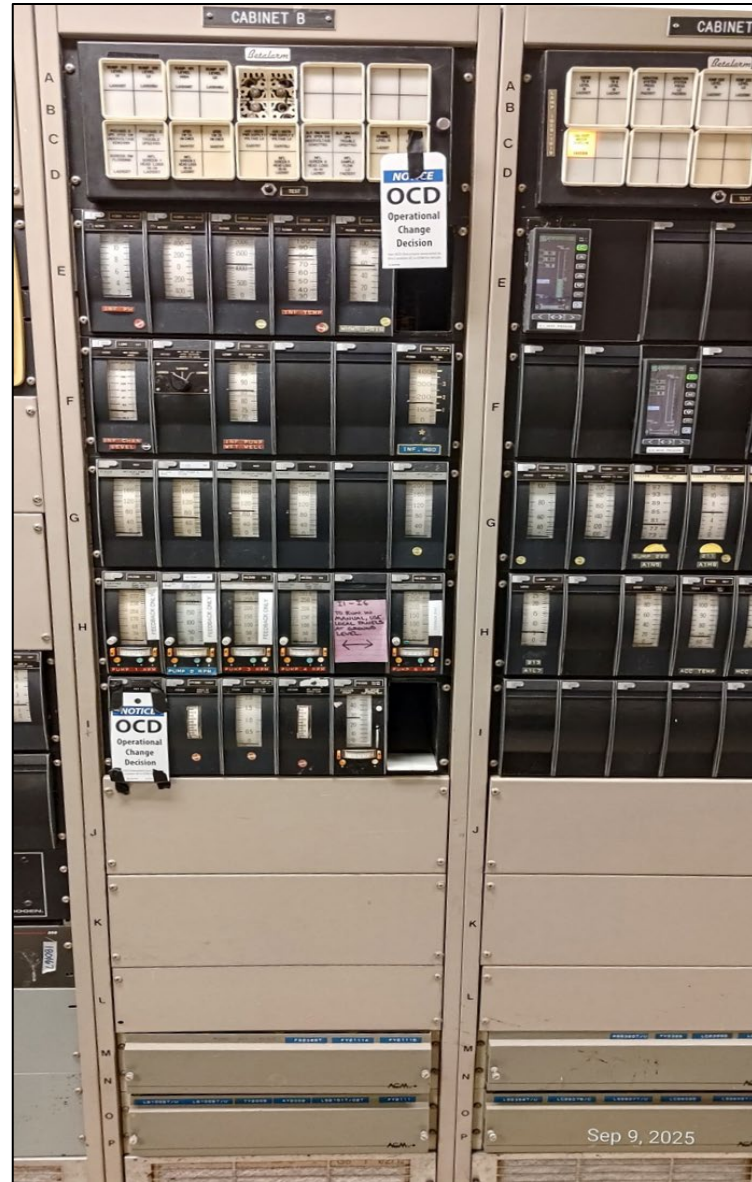
PHOTO 4 ALARM PANELS AND ANALOG CONTROLLERS
