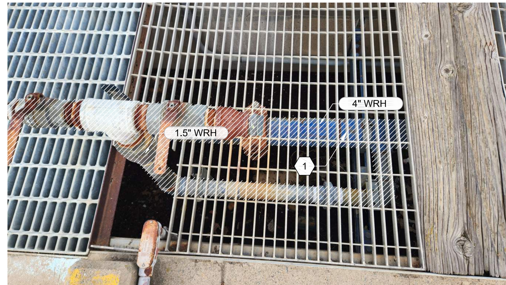
B6 PHOTO 31D101 3US45 - UTILITY STATION PIPING AT COLUMN 9&10 DETAILS. (TYPICAL FOR COLUMNS 5, 14, 18&19, AND 23)
