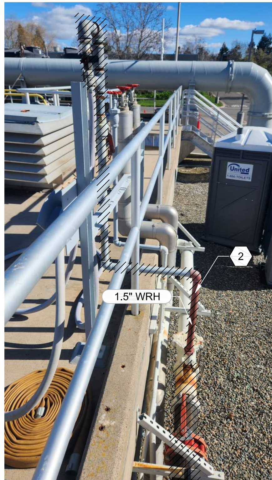
U1 PHOTO 31D101 3US19 - MAIN HEADER UTILITY STATION
