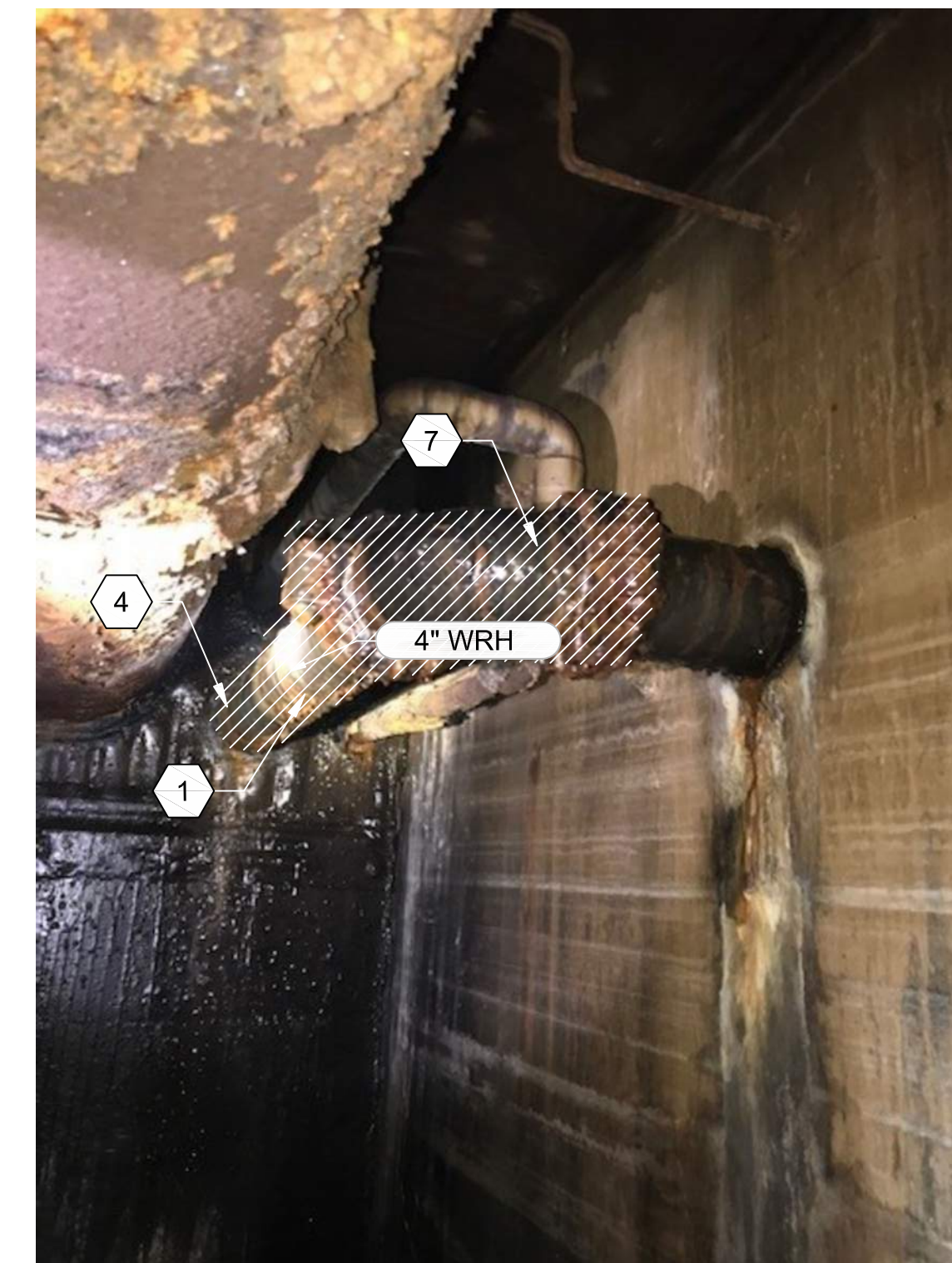
H6 31D101 PHOTO WRH MAIN HEADER AT NORTH SIDE OF PRIMARY TANKS
