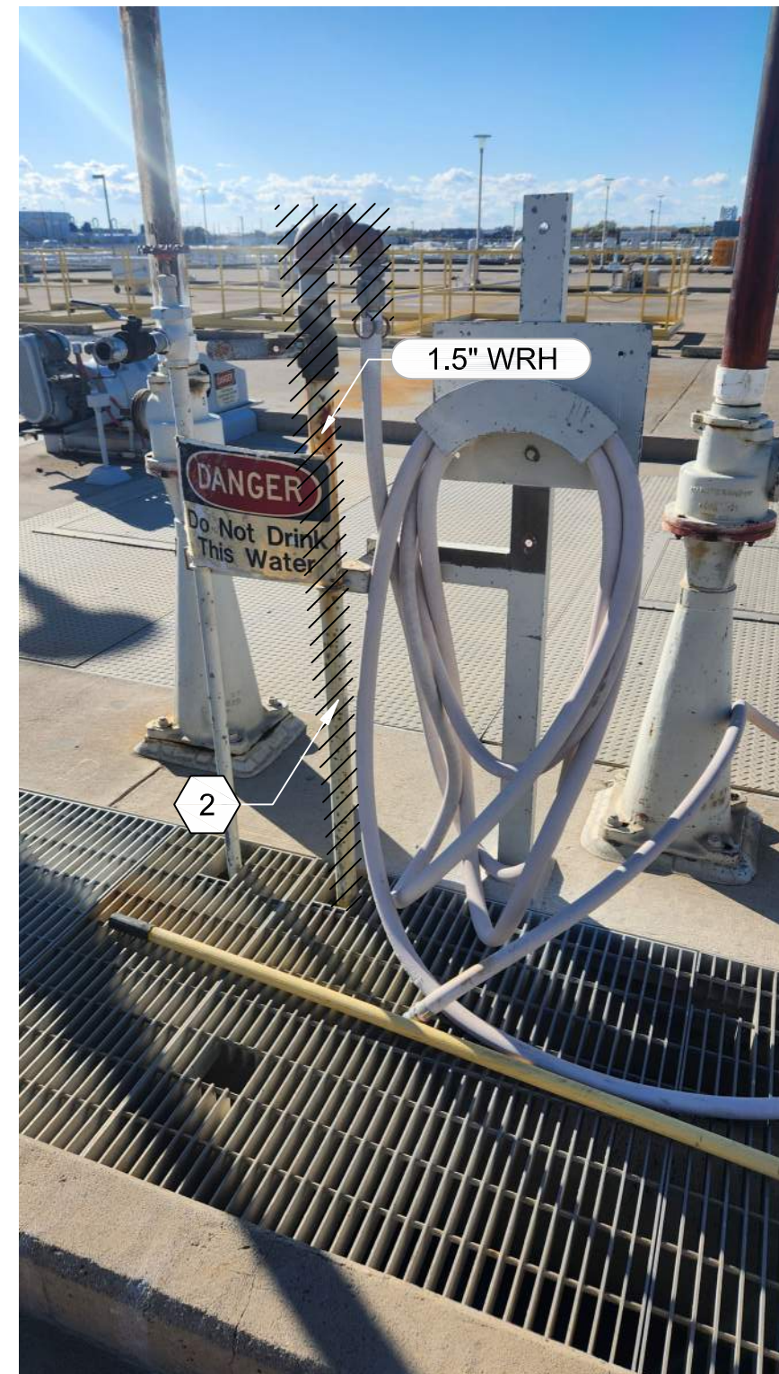
U2 PHOTO 31D101 3US17 - MAIN HEADER UTILITY STATION. (TYPICAL TO 3US13 AND 3US18)
