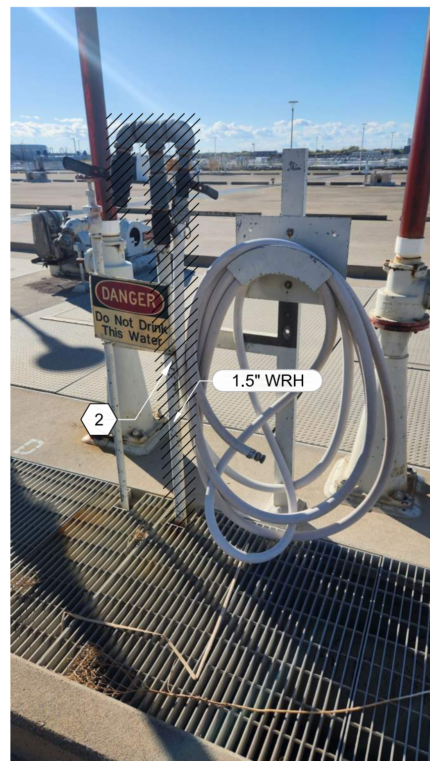
U4 PHOTO 31D101 3US16 - MAIN HEADER UTILITY STATION. (TYPICAL FOR 3US14, AND 3US15)
