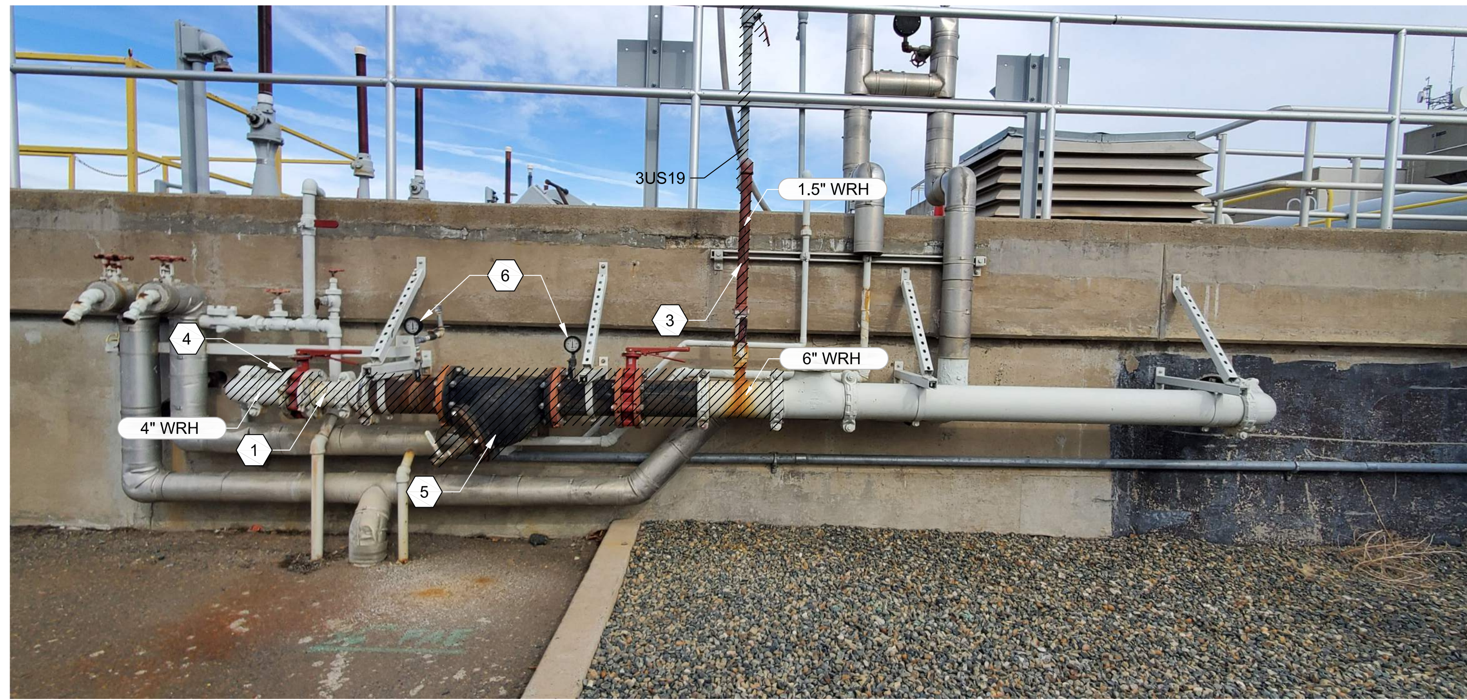
H1 31D101 PHOTO WRH MAIN HEADER AT SOUTHEAST OF THE PRIMARY TANKS
