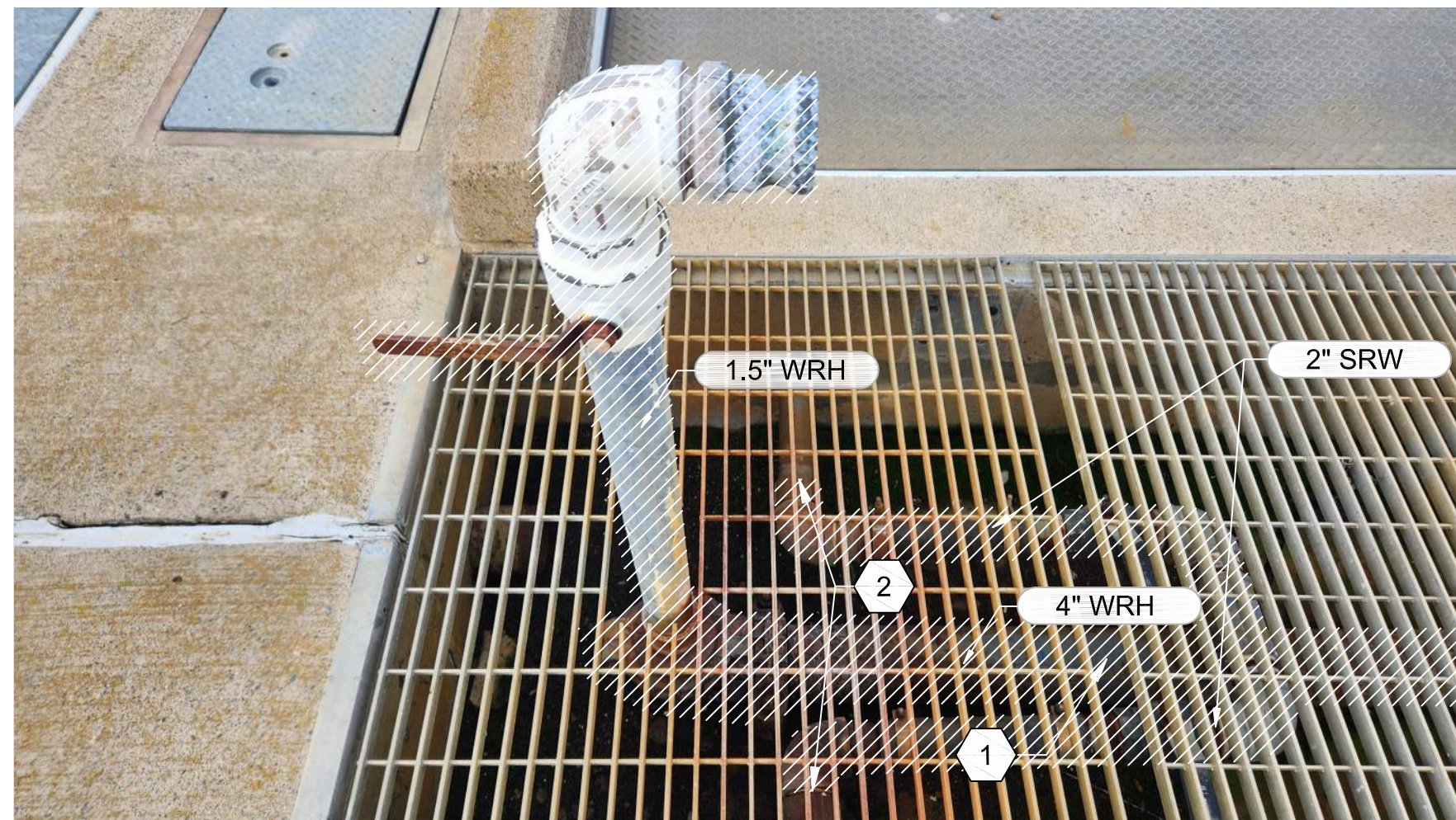
B7 PHOTO 31D101 3US44 - UTILITY STATION PIPING AT COLUMN 14 DETAILS. (TYPICAL TO COLUMNS 18&19 AND 23)
