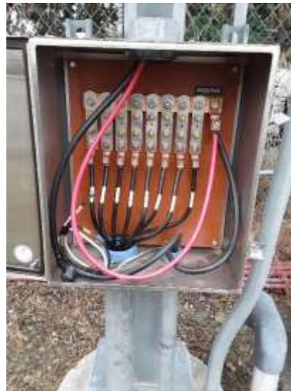
Photo 5-2. N24-CPNL0033A Anode Junction Box
