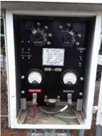
Photo 5-1. N24-CPNL0033A Rectifier Panel
