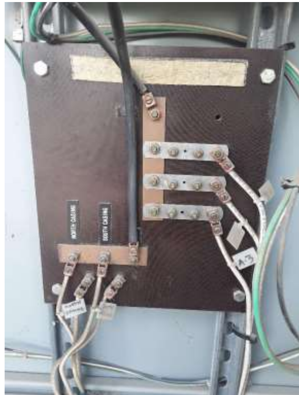
Photo 5-4. N52-CPNL0001A Anode Junction Box
